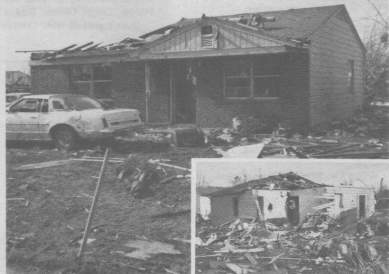
PATH OF DESTRUCTION —Every room of the home of Church members John and Minnie Spencer sustained damage when tornadoes swept through eastern Arkansas Dec. 14. Inset: The back of the Spencers' house. [Photos by Mark Cardona]
